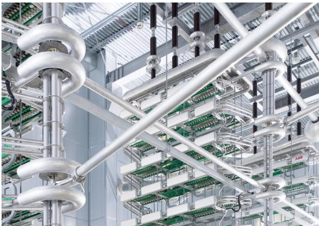
Valve Hall. Courtesy of ABB
